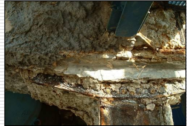
Corrosion beneath concrete
